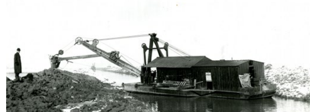
Dredging the Surplus Canal on the Jordan River, June 1913. Used with permission, Utah State Historical Society.
